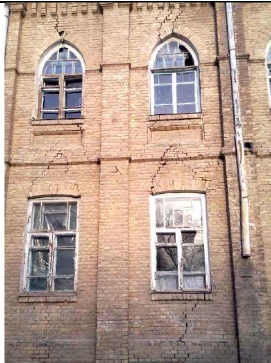
Fig. 10. A fragment of the western end wall of the building; dangerous settlement cracks are present, and restoration using historical masonry materials is recommended.
