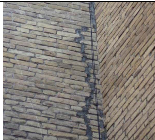
Fig. 8. Sealing a crack with cement mortar reduces the architectural value of the building.
