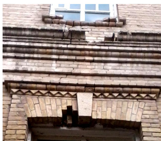
Fig. 5. A fragment of a building wall made of ornamental masonry with significant cracks requiring restoration using historical materials.
