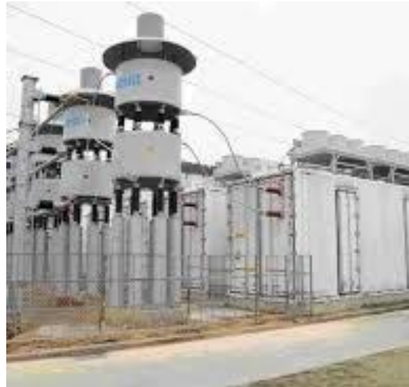
Fig.1. General view of the STATCOM device
